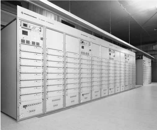
Fig. 31.21. DVB-T transmitters Olympic Tower Munich; manufacturer's photo, Rohde&Schwarz.
