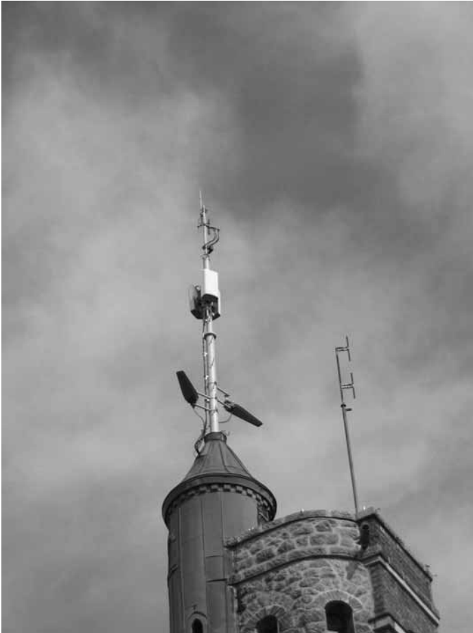
Fig. 31.38. Practical example of a translator or gap-filler site; the 2 (log periodic) receiving antennas are located in the lower part of the extended pinnacle of the tower, the 3 transmitting antennas (8-element bays) are located in its upper part
